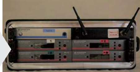
Sennheiser antenna splitter and receivers
