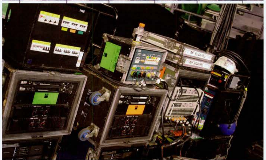
Assorted JPJ amp racks for Surround arrays
