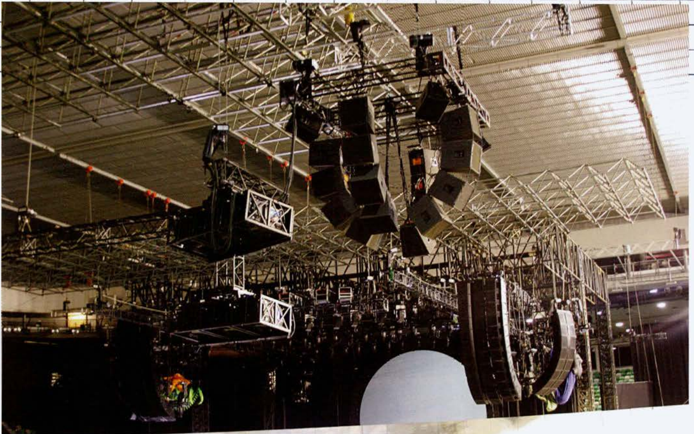
Surround cluster, several projector carts and main system
