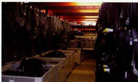
Neat cable street
