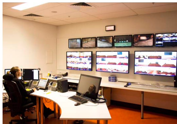
| MCEC TECHNICIAN LORA THOMPSON IN THE MASTER CONTROL ROOM
