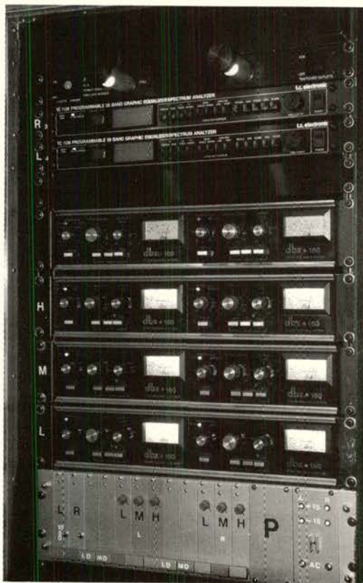
F.O.H. drive rack, with the T.C. Electronics Digital Equalisers at top, DBX 160 limiters, (still the best for the job), and proprietary processor at the bottom.
