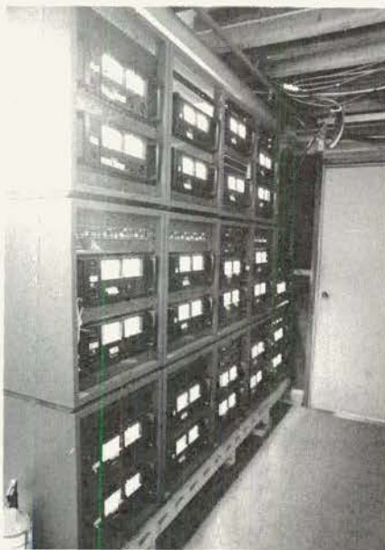
Part of the amp room- 61 Yamaha amplifiers drive this system.
