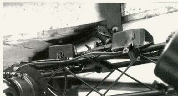
Who is responsible for the wiring? The first installer had the job wired then pulled it out. In any case, these terminal blocks atop the lighting truss show signs of hasty installation.
