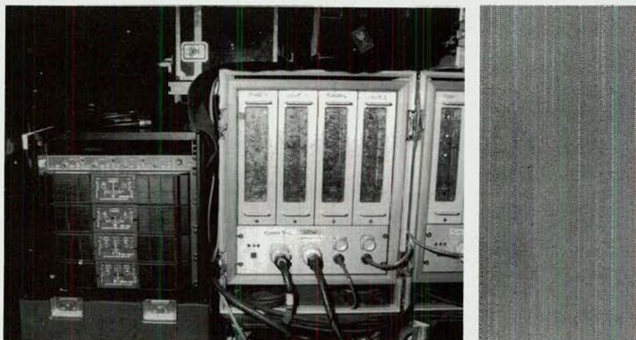
Ocecnia's racks at right, compulsory BSS/Turbo rack for Flashlights at left.
