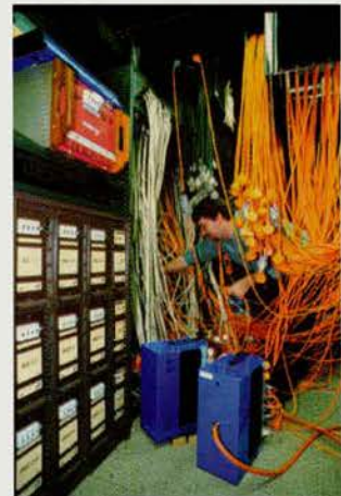
Dene Jones at the patch panel of the Academy Theatre
