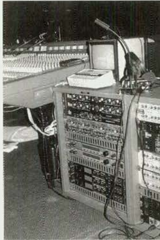
Racks, Lexicon processors centre.
