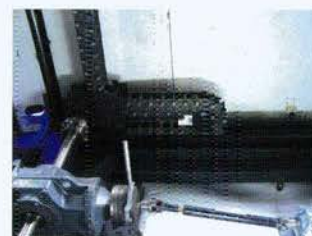
Serapid lift detail. Marcus stands under the orchestra lift (top), and this is how the self climbing chain works. Neat, huh?
