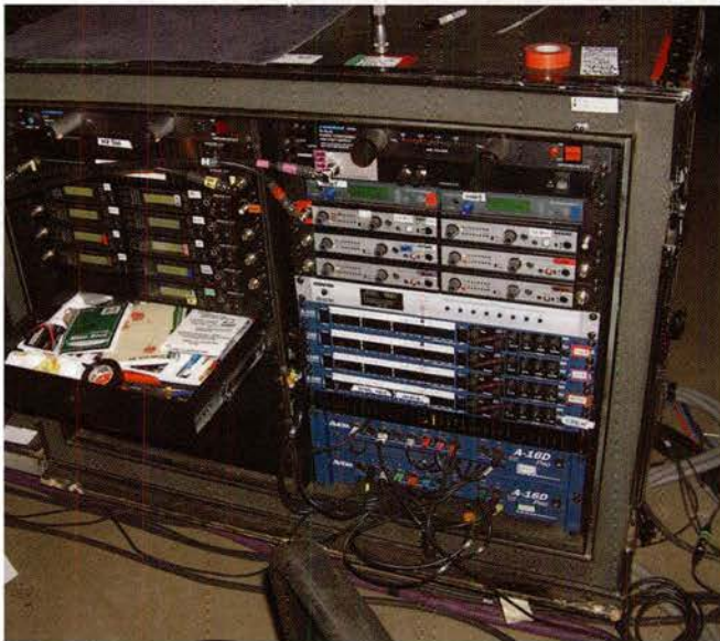
Wireless rack, and Aviom units (above).
