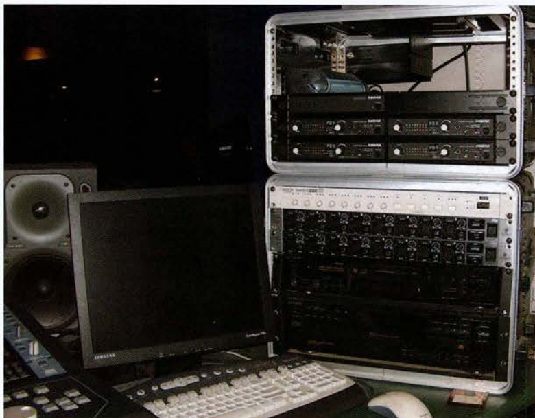
FOH racks with some analog to digital (a-d) converters, Sony MD and CD decks, and Shure PSM transmitters at top.
