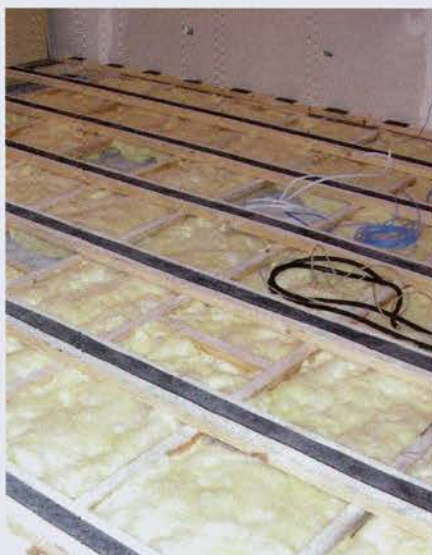
First run of floor joists sit on rubber, second run stabilise them. Rubber on top, then particle board, then floorboards
