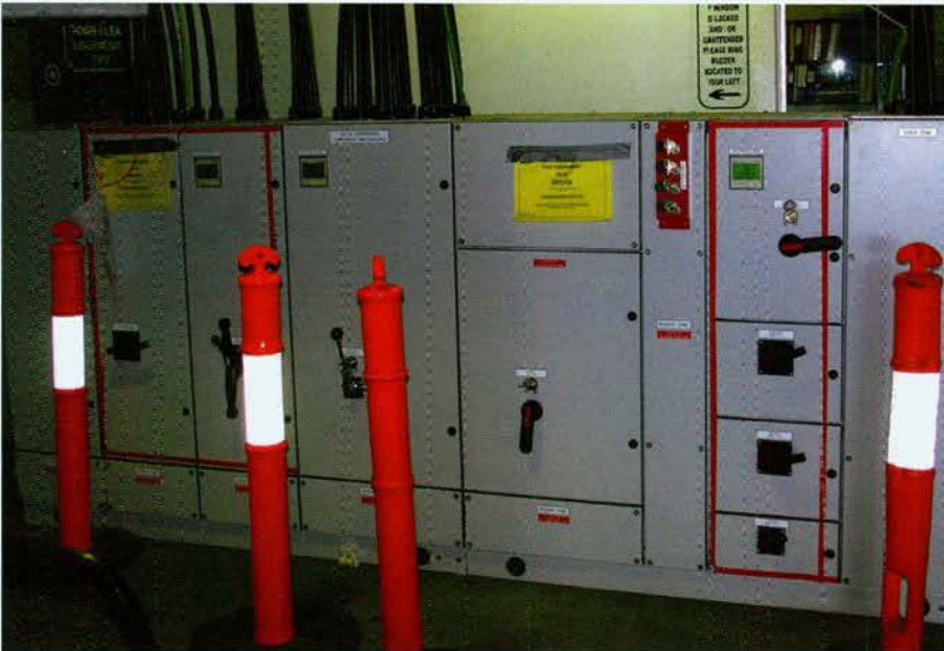
One of 3 Power Change Over - 650Camps per phase.
