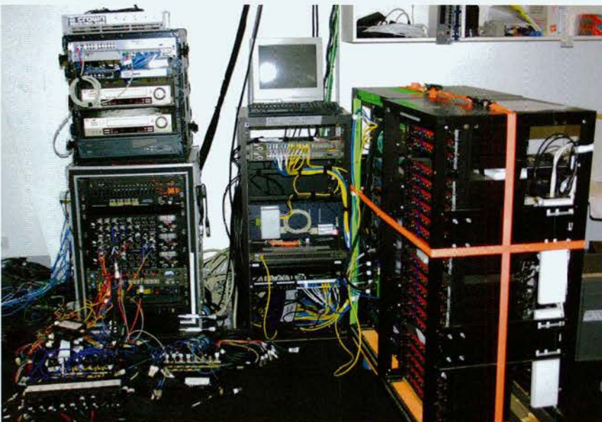
Control Room Audio and LX data.
