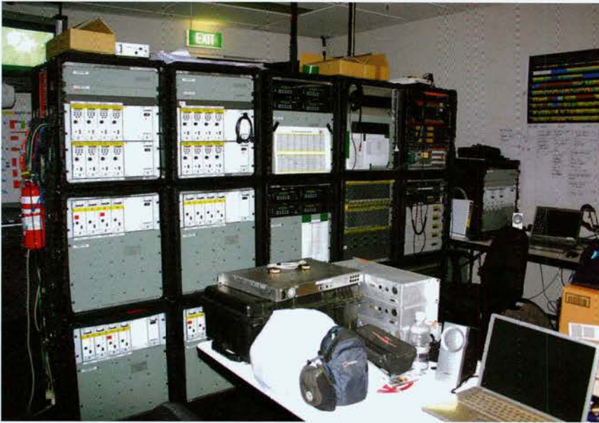
Communications radio racks.
