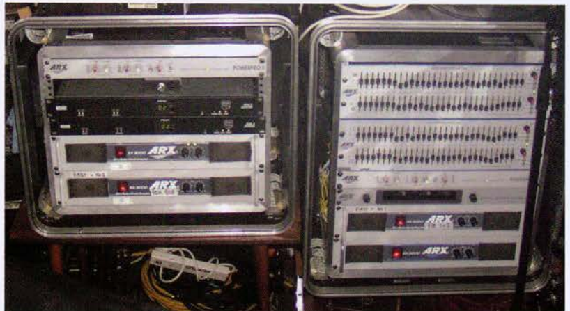
Backstage space is at a premium. Note EPA compulsory level sensing limiters from Rane.
