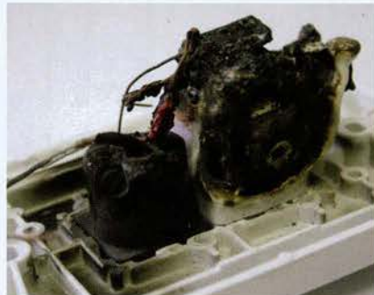
Fire in the hole! What's left of the offending dimmer switch.
