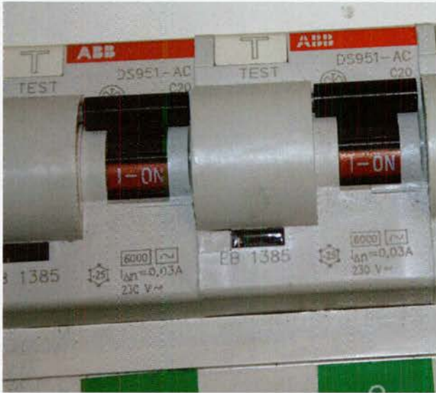
RCCBs used instead of a single 3 phase RCD.
