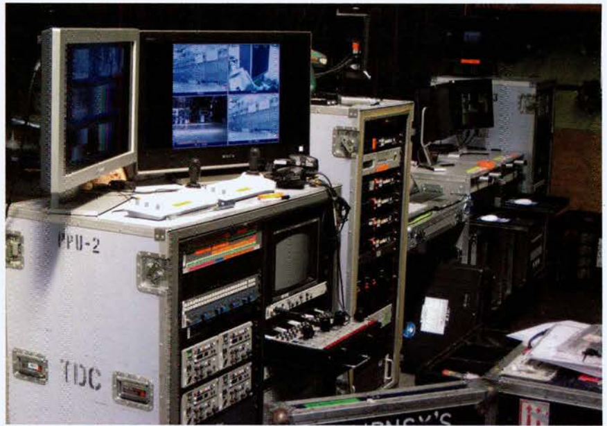
The whole show fits into 6 racks and one table backstage – with redundancy!
