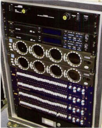
Drive racks include redundancy for everything
