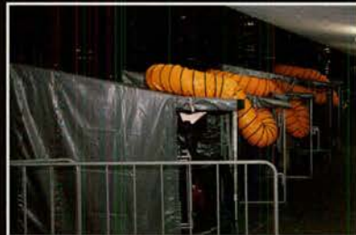
Even in midwinter, the fourteen Christies aimed at the Opera House need some serious cooling
