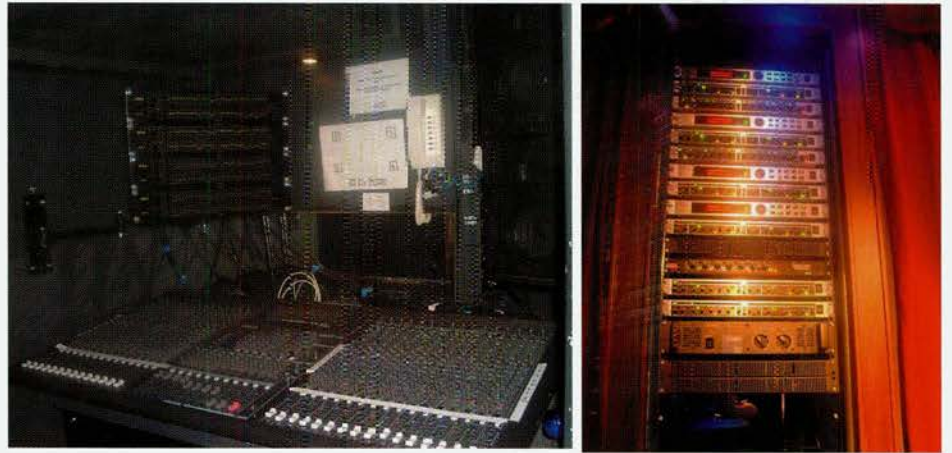
Stage monitor console, 8 sends, tucked in a side stage passageway. Processing rack (right) is part of the stage design.
