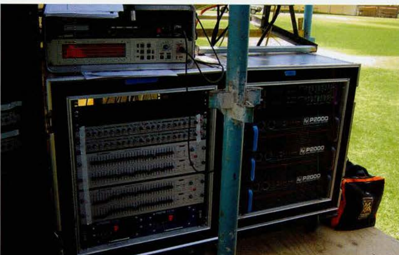
Console power supply with insert and FOH EQ's, plus delay amps and system drive in adjoining rack
