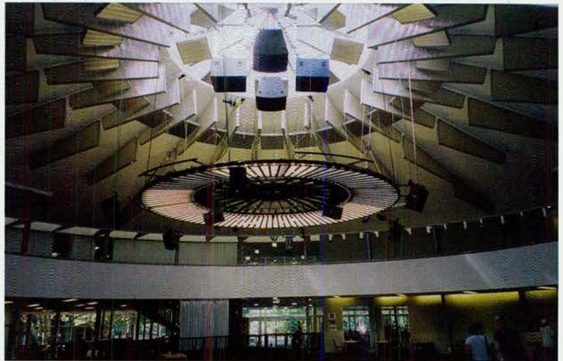
Four Meyer subs flown facing down, above the circle of UPA-1P's - six facing out, and two facing down. More UPA's are placed on time delays through the venue.
