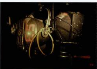
Patt 23 with dangerous asbestos cable (left) and the black PTFE cable (right)
