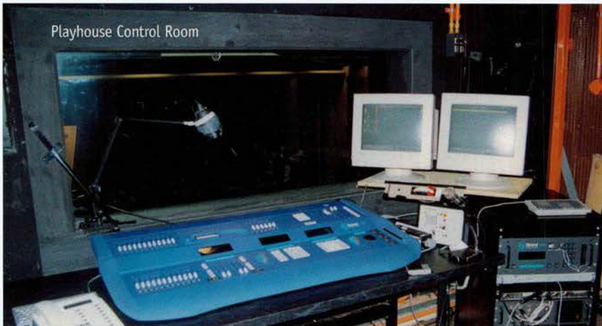
Drama Theatre Control Room
