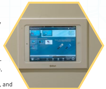
>> Crestron control via iPad
