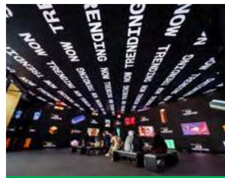
Now Trending is served by L-Acoustics X4i installed at ground level under the screen, SB10i hidden in the floor grate, and with 5XT and Syva Sub suspended around the perimeter of the room at transom level
